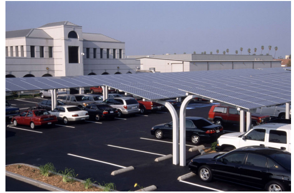
Photovoltaics over parking area APC Schott
